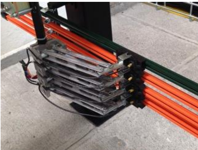
Insulated Conductor Bars and Collectors
