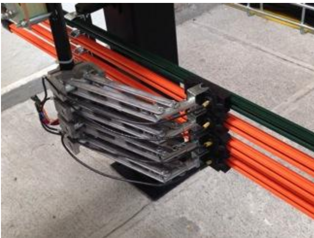
Insulated Conductor Bars and Collectors
